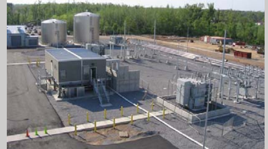
Two-section, electrical equipment enclosure with 480V switchgear, MCCs, battery & UPS system. Location: Paducah, Kentucky
