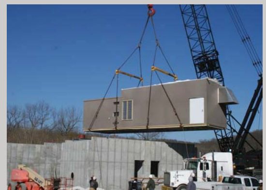
Four-section, modular enclosure with medium voltage control room. 28' wide X 47' long X 14' inside height. Location: Joplin, Missouri
