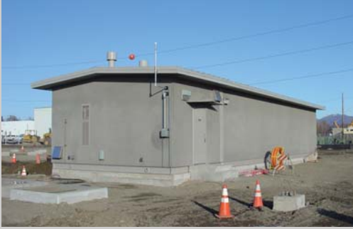
Two-compartment, relay panel enclosure with standing seam metal roof. 21' wide X 64' long X 11' inside. Location: Anchorage, Alaska
