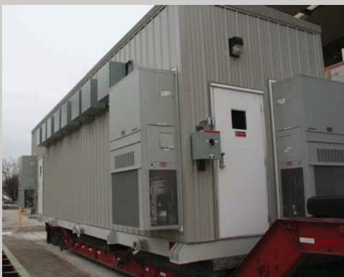
Electrical equipment enclosure with steel exterior walls. Location: Savannah River Nuclear Site, South Carolina
