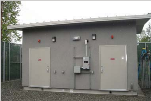
Substation control enclosure with standing seam metal roof. Location: Anchorage, Alaska
