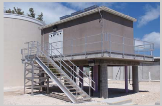
Utility enclosure designed for 150MPH wind load with standing seam metal hip roof and equipment hatches. Location: Duck Key, Florida
