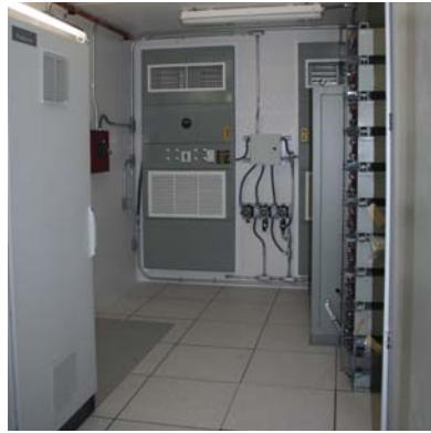
Remote instrument enclosure with 12" deep computer floor and H2S filtered HVAC system.
