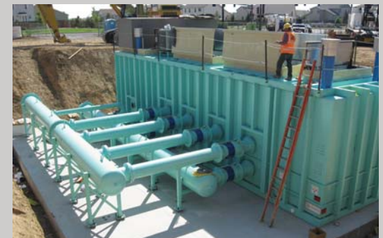
Below grade steel electrical equipment enclosure for pump control switchgear. 14' wide X 51' long X 11'-9" inside height Location: Thornton, Colorado
