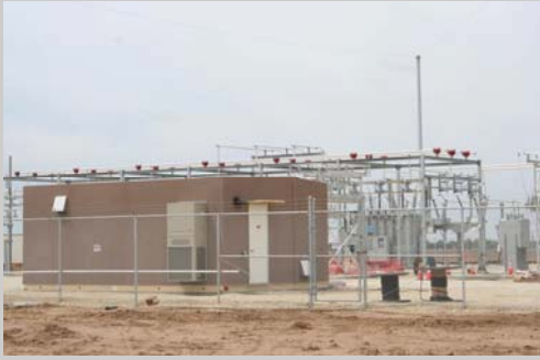
Relay panel enclosure. Location: Wichita, Kansas
