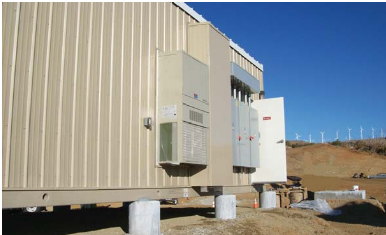
Wind farm control enclosure with relay panels, UPS system and server room. Location: Kern County California
