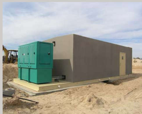
Factory installed & tested diesel powered stand-by generator enclosure. Aluminum base floor structure. Location: Lake Havasu, Arizona
